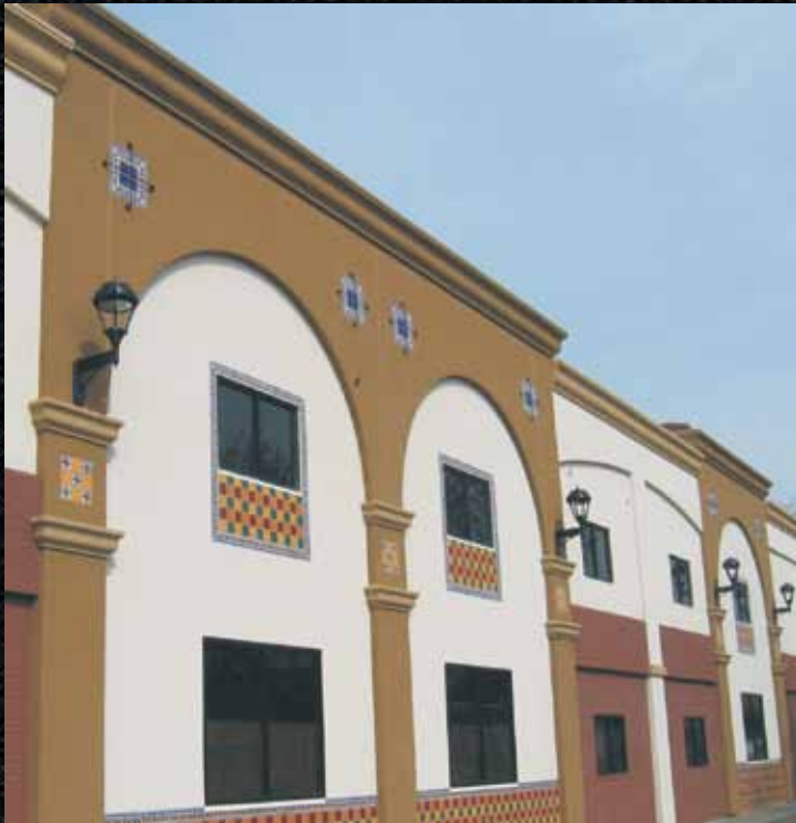
BAROQUE 7, CINNAMON, YELLOW, COBALT, AND GREEN. MEDICAL BUILDING EXTERIOR RENOVATION. SACRAMENTO, CA
